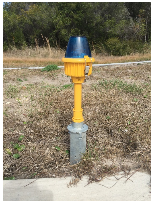
Figure 2.16. Medium Intensity Taxiway Edge Lights
