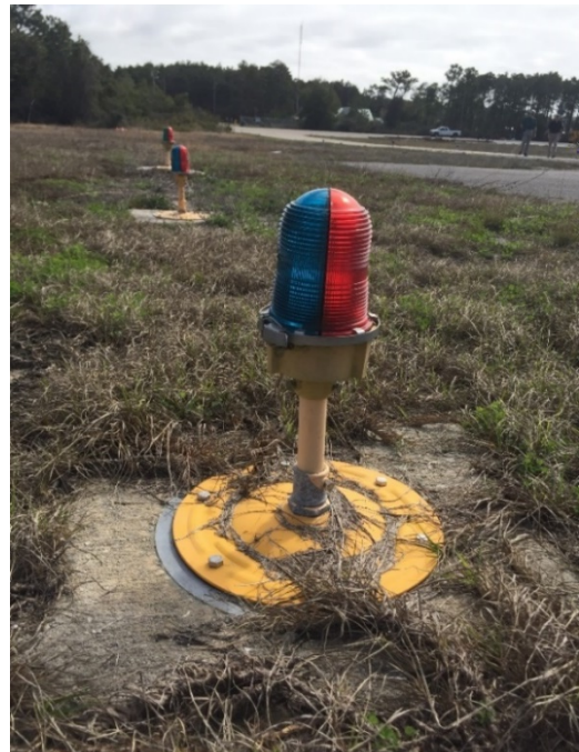
Figure 2.13. Runway End Identifier Lights
